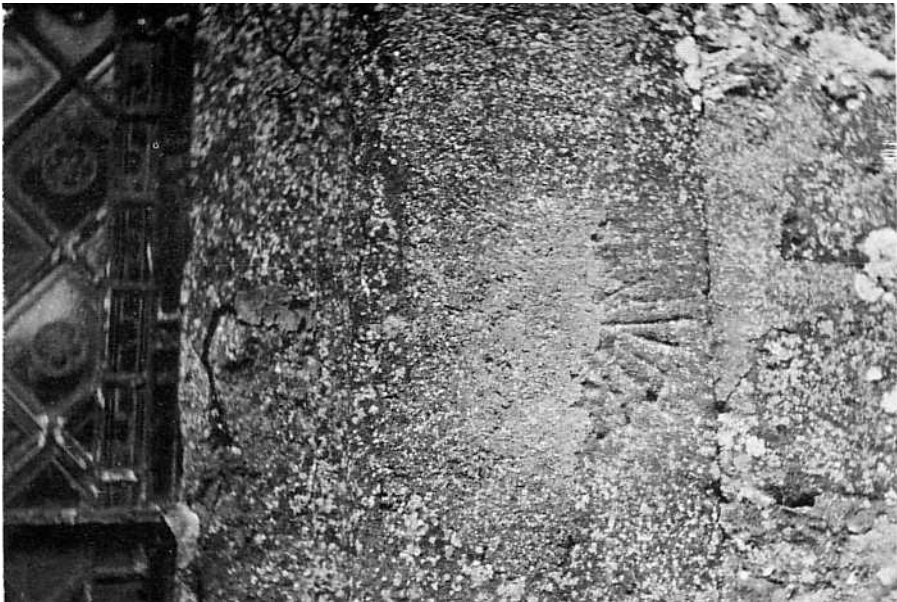
Figure 3. Partial obliteration of dial by restoration of stonework with mortar. Duns Tew, Oxon.
